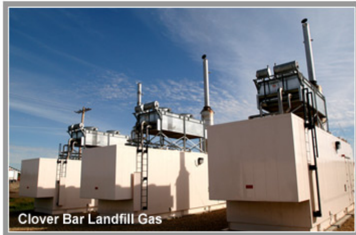
Figure 5. Clover Bar Landfill Gas Generating Units
